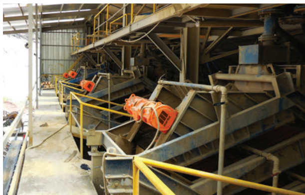
Figure 1 – Screen vibrators are wear parts, so ergonomic access is important for workplace safety.
