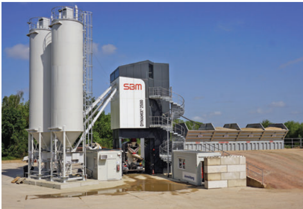
Bridging mobile and stationary concrete production, the SBM DYNAMIX 2500 also meets high demands regarding plant design. (Photos: SBM)
