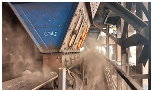
Figure 3 - Dust can create serious issues at transfer points. Containment is key
